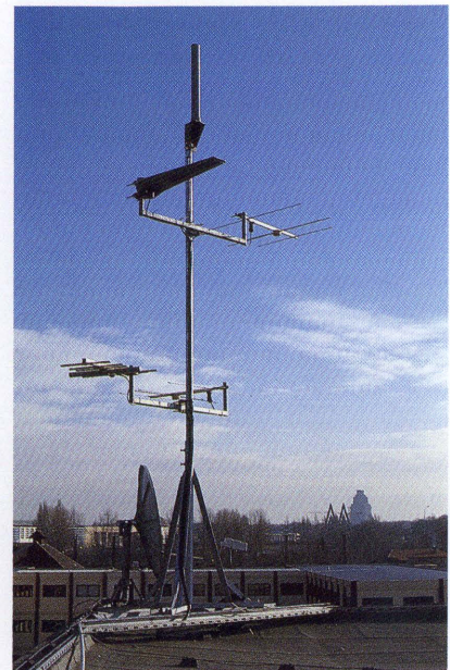
FIG 1 Rack layout of TS9965 for single station and antenna of radiomonitoring system at Mitteldeutsche Rundfunk in Leipzig Photo: author
